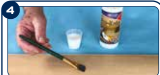
4 Apply an initial coat of Eze-Kote resin and allow it to dry.
